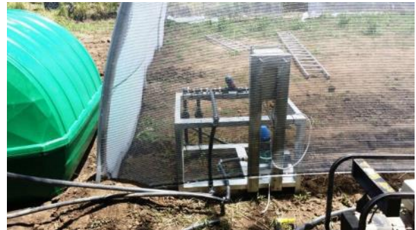
ABOVE: Irrigation scheme constructed by Greener Solutions and the Lima engineering team.
